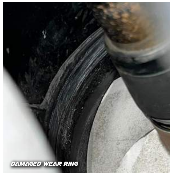
DAMAGED PUMP IMPELLER
